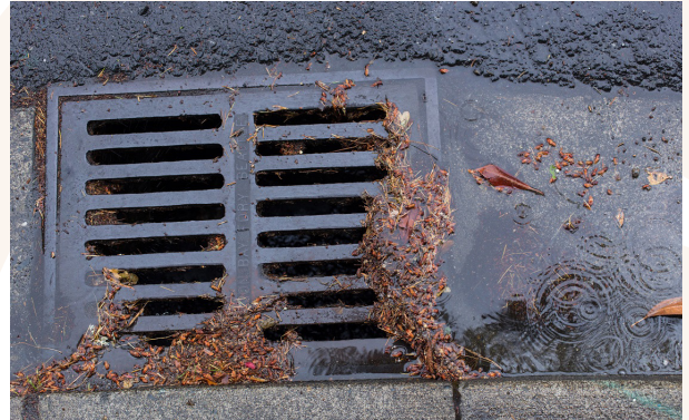
Street sweeping is an important part of keeping drains clear and preventing flooding.
