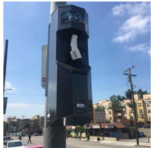
Example of an EV charging station mounted on a public utility pole in Los Angeles. Photo credit: Barry Lank
