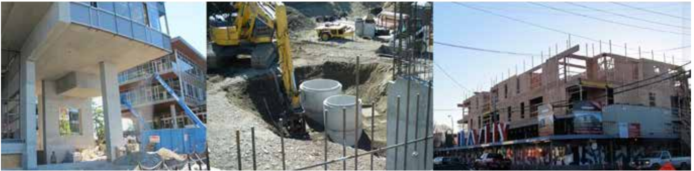
26.6.5 Pollution management protocols (including sedimentation and oil- removal), as well as recycling programs should be followed during demolition, excavation and construction of the project.
