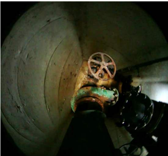
Figure 7 - Uganda PS - Pump 1 Bottom Level (2)
