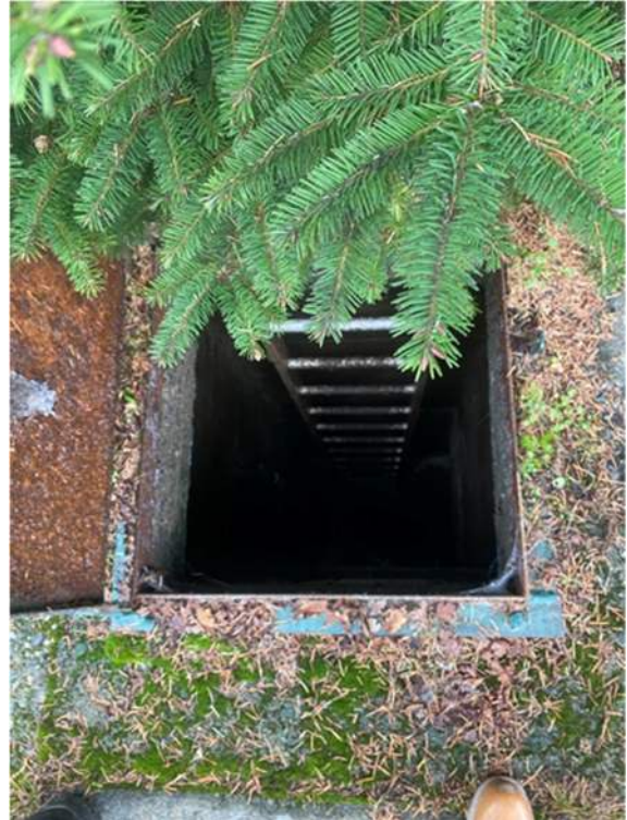
Figure 14 – Uganda PS – Wet Well Entrance
