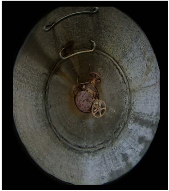
Figure 12 – Uganda PS – Bypass Chamber
