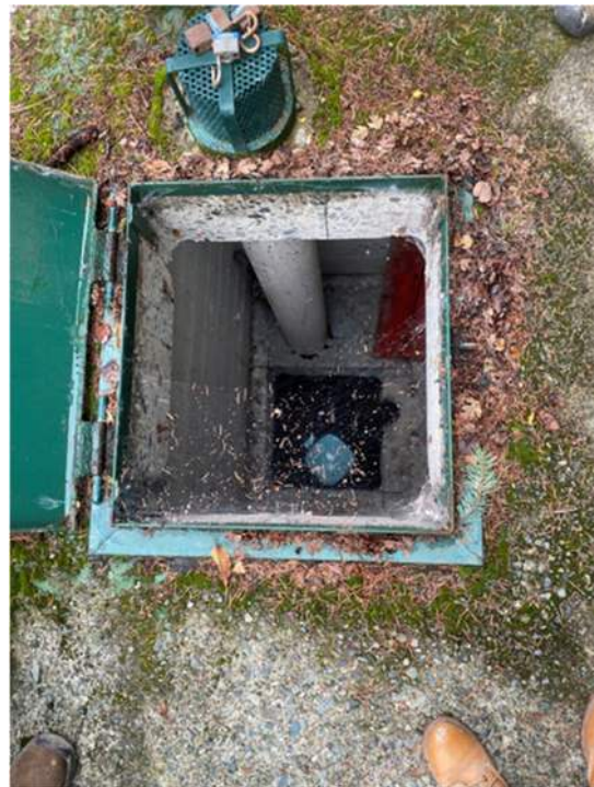
Figure 4 - Uganda PS - Pump 1 Entrance
