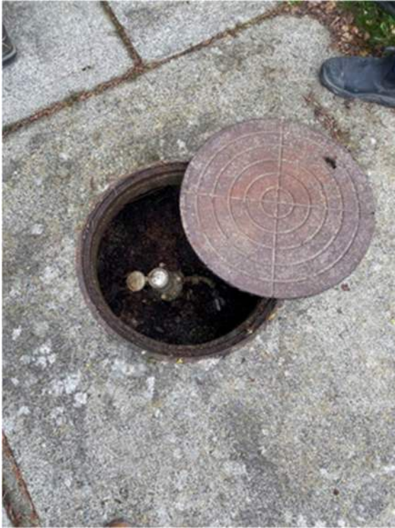
Figure 13 – Uganda PS – Water Vault
