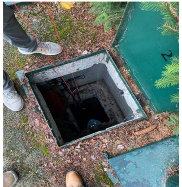
Figure 8 - Uganda PS - Pump 2 Entrance
