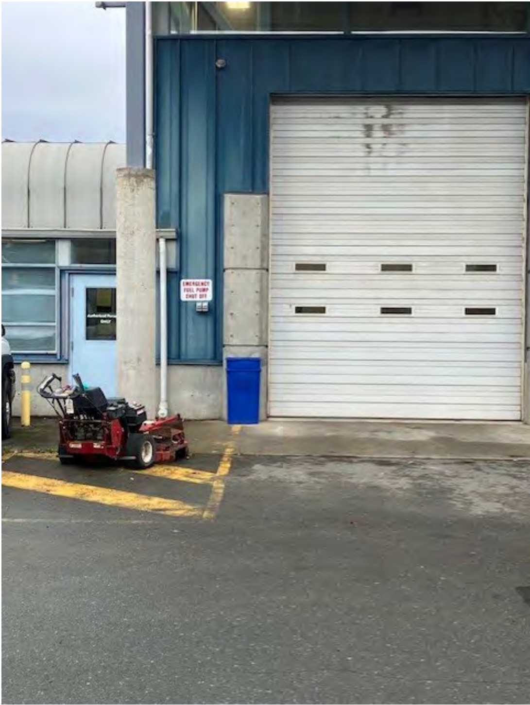
Figure 6 Existing fuel pump shut off on building wall.
