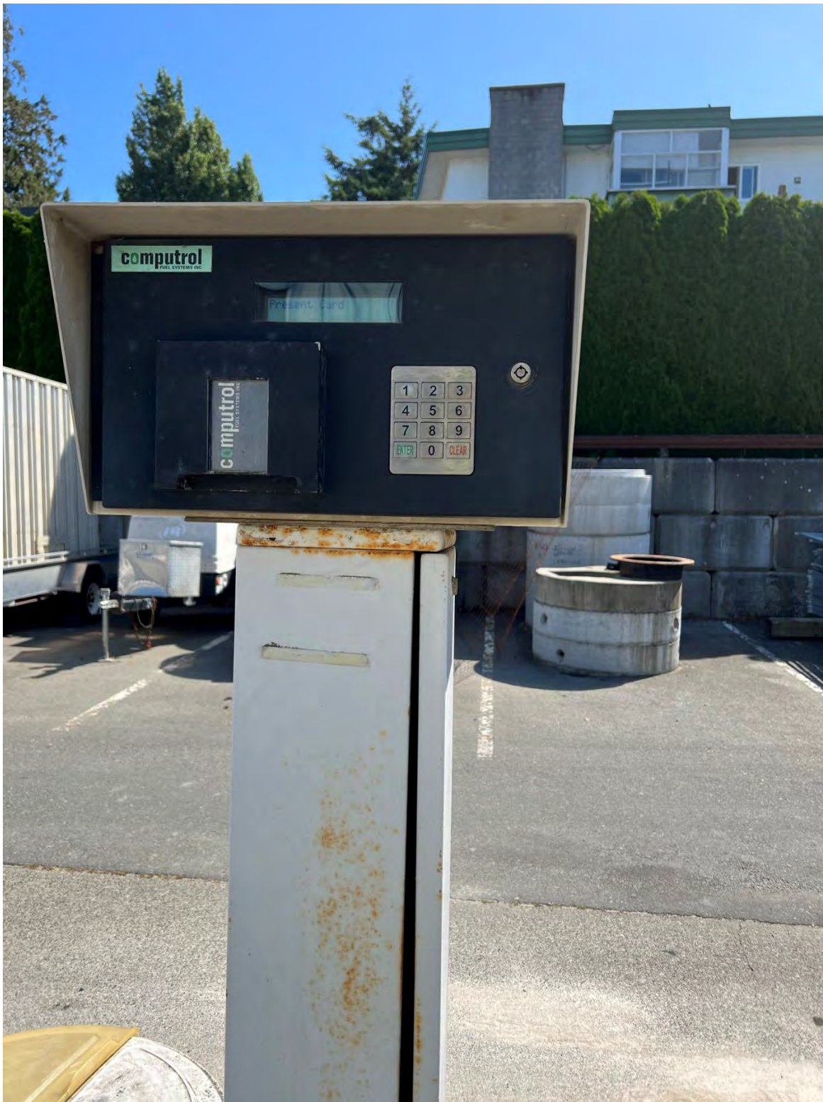
Figure 7 Existing card reader to be removed once new card reader has been commissioned.
