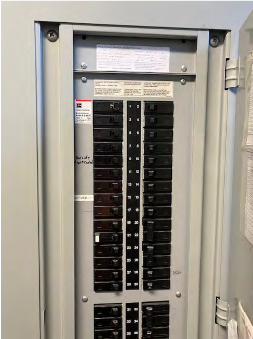
Figure 8 Electrical panel near emergency shut off switch with spare capacity for power to new fuel pumps and controls.
