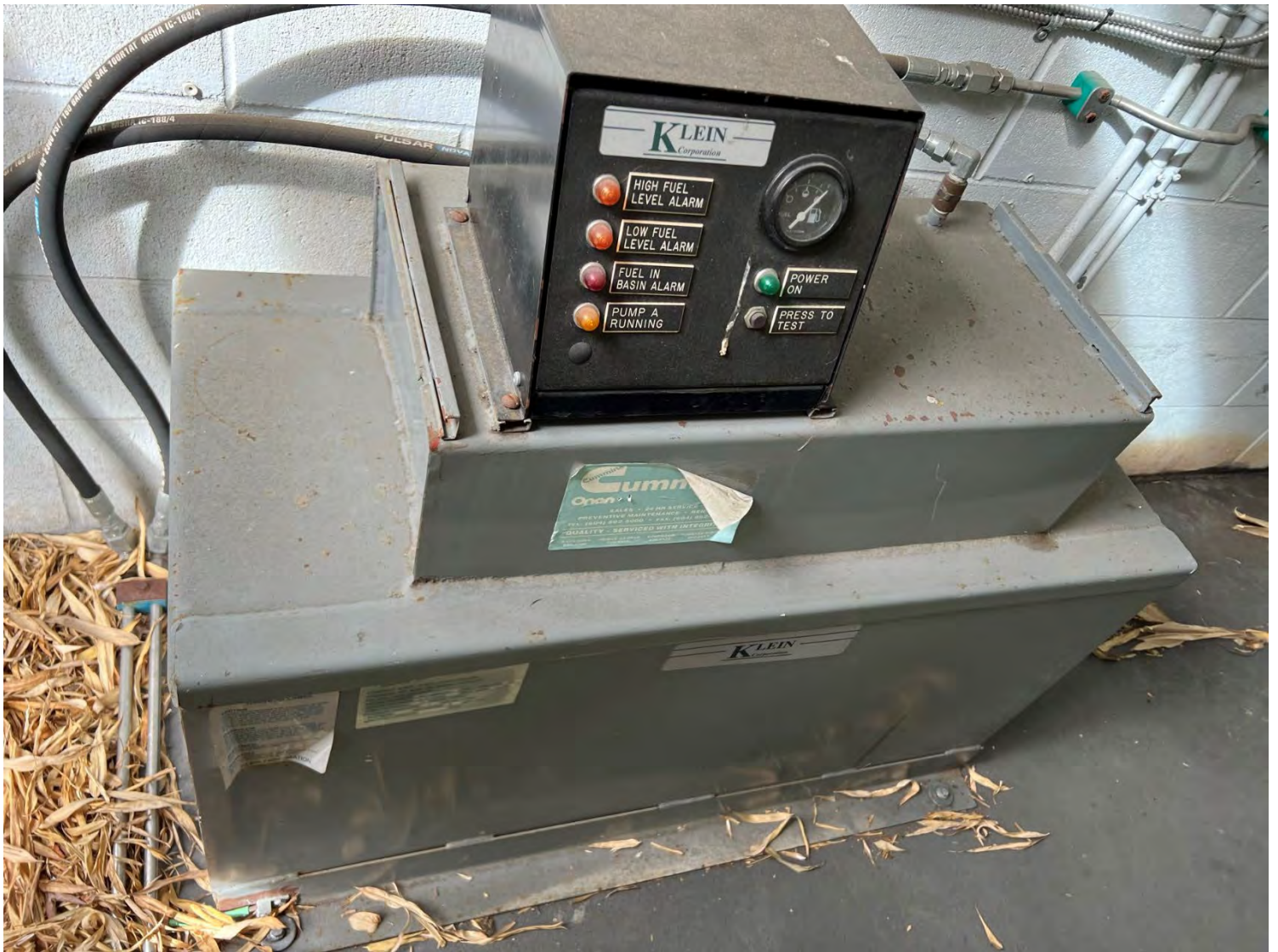
Figure 4 Generator day tank and alarm panel
