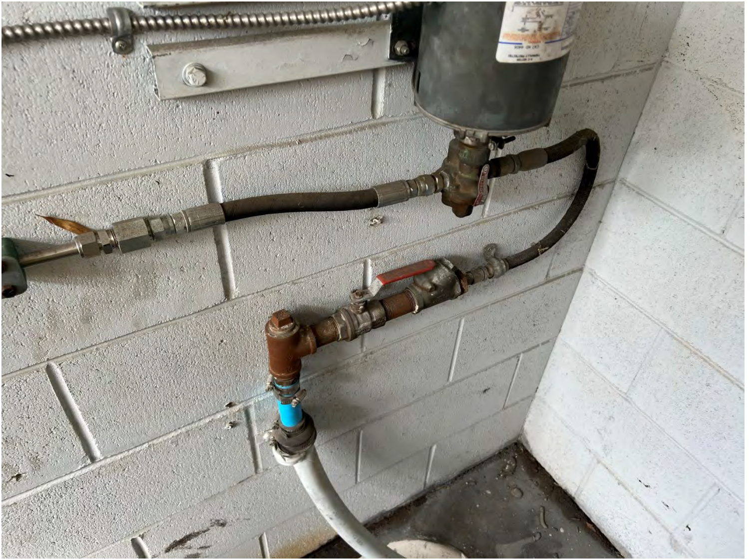
Figure 3 Emergency Generator suction pipe through floor connected to the suction pump that filles the day tank
