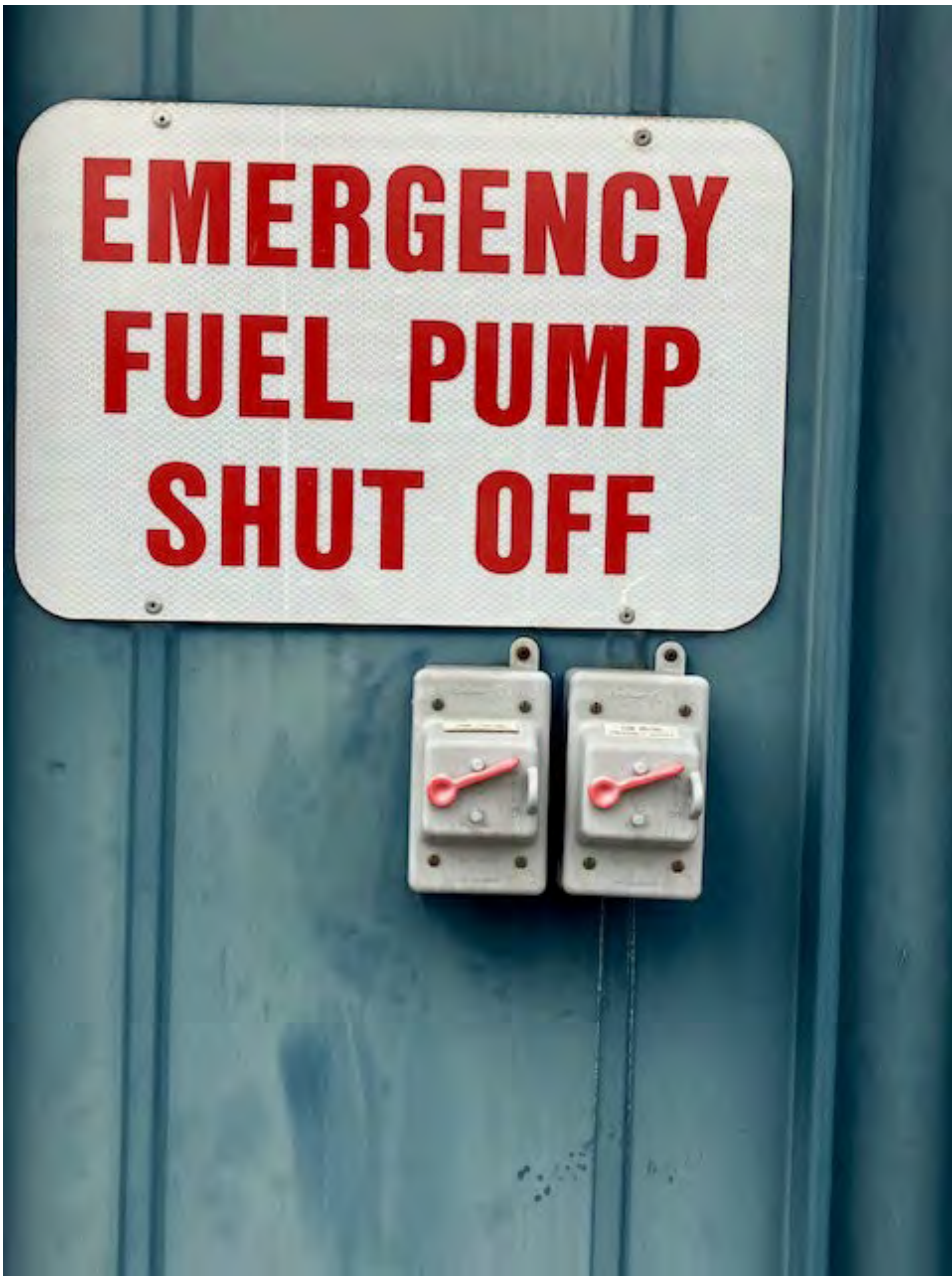
Figure 5 Existing fuel pump shut off to be replaced with a new one for the new fuel tank
