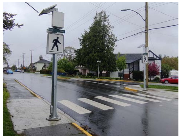
New Rectangular Rapid Flashing Beacon (RRFB) crosswalk on Lyall St. at Paradise St.
